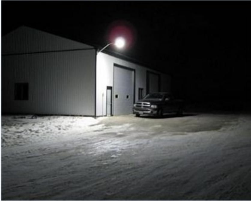
Retrofit LED street light 60w
